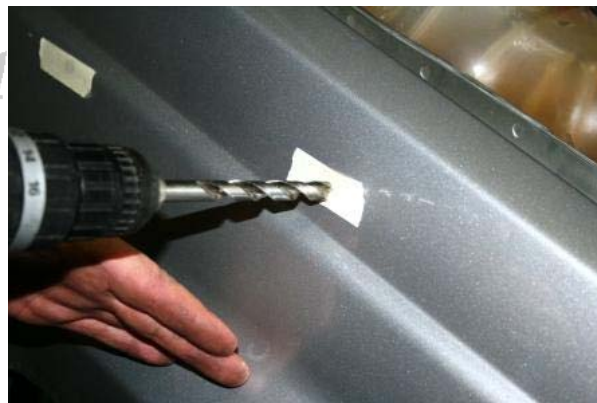
3.39 Cover with masking tape 3.40 Using a 10mm bit, drill the 5 fixation holes (not the snorkel hole)
