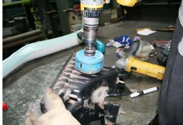
3.20 Using the 90mm hole saw, drill at SLOW speed a 90mm hole in the air box
