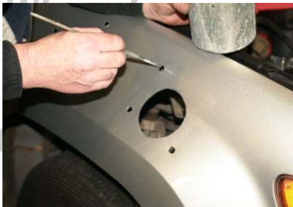
3.45 Paint ALL raw metal surfaces with Zinc rich primer (7 snorkel fixing holes, 1 air intake hole including inside panels)
