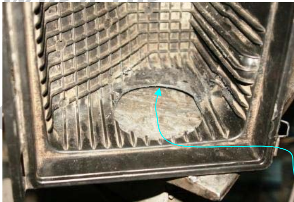
3.15 Grind away the bottom ribs inside the air box to achieve this result.
