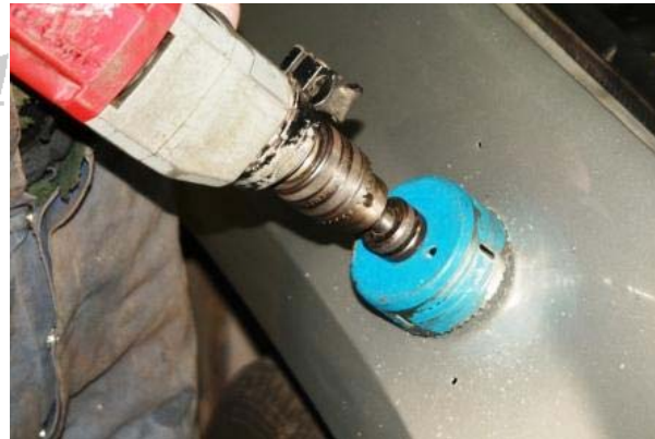
3.42 Using the 90mm hole saw, drill at LOW SPEED the snorkel hole
